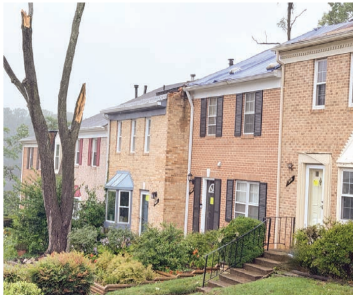
Yellow placards line doors of damaged homes indicating use is limited to safe parts of the structure or for temporary clearing of belongings after county inspection.
