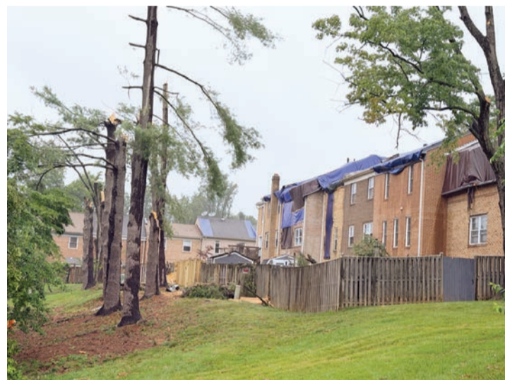
Blue tarps dot roofs to protect damaged houses.
